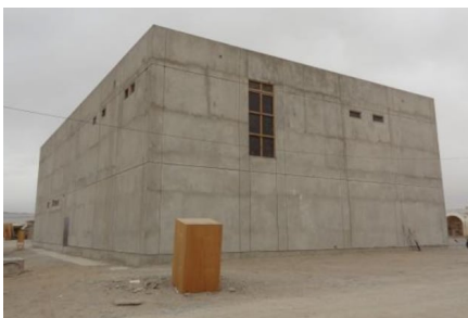
The unfinished headquarters for a Special Forces base in Kandahar. (Courtesy of SIGAR)
